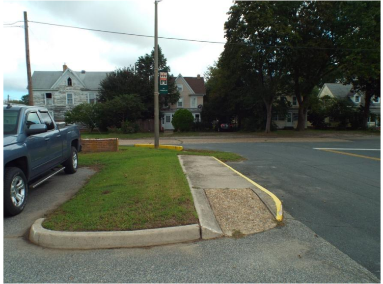
In the picture above you can see an abrupt stop to the sidewalk with no curb cut available on one side.
